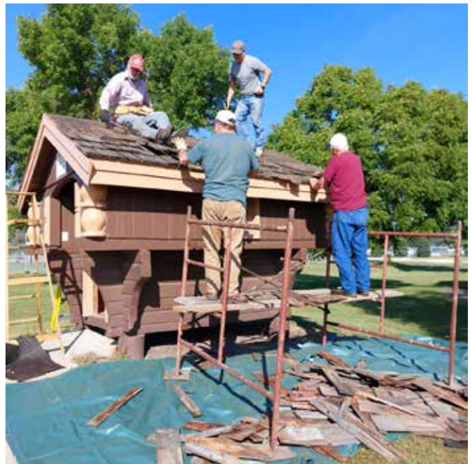
(Above) The small stabbur in the Sons of Norway Park in Bismarck needed a new roof. Tom Marple, Mark Holkup, Jerry Saude, Ken Lien, Lavrans Johnsgard and Claudia Berg spent a Saturday reroofing, finishing just as the rain began falling
